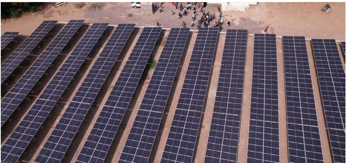
A 610-kilowatt solar-powered station and an electrical grid were installed to ensure uninterrupted water supply. Photo: Al-Twasul
