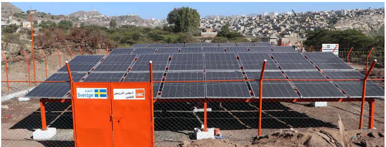
Solar power system installed by NRC for the water scheme of Al-Osa Asabeh in Taiz governorate. Photo: NRC
