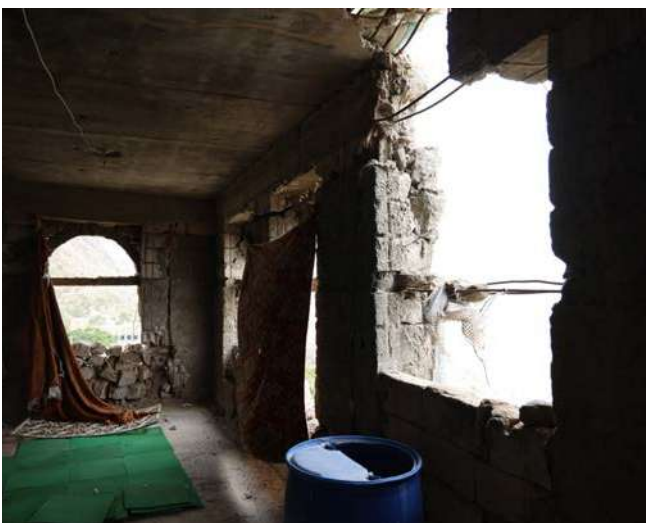
Waseem's house before intervention. Photo: NMO
